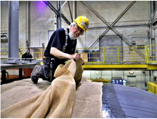
Jumping ahead to the "A" end, Quasimodo, temporarily neglecting his bell-ringing duties, and having applied a strip of contact cement to the bonnet deck, here deploys the burlap underlayment. (Photo by Jim Houston)
