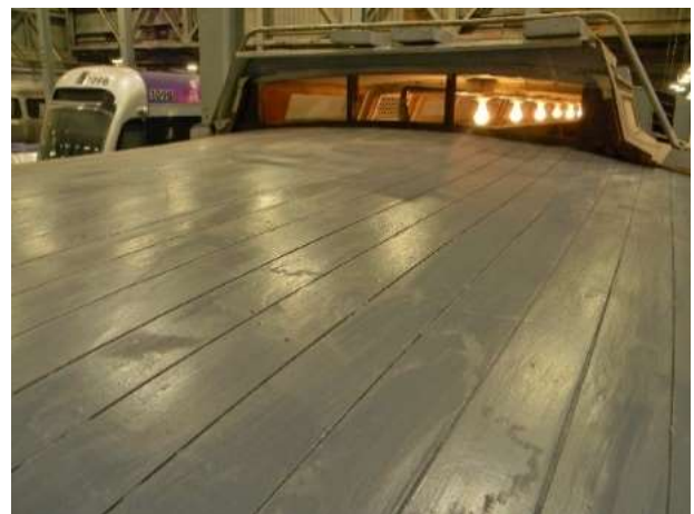
One of the first tasks at hand was to enamel the sheathing of the bonnet roofs in order to protect the ancient planks from any errant moisture that might infiltrate the canvas cover to come.
