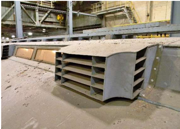
Hurried temporary mounting of all eight ventilators back in 2017 now required a more permanent solution.
