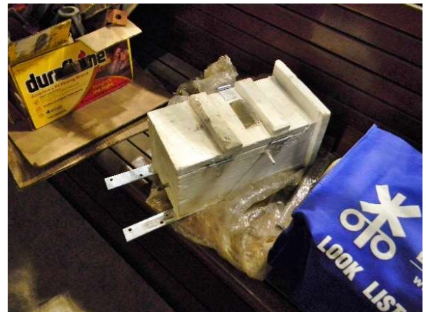
The lightning arrester, cosmetically restored by Tony, awaits installation.
